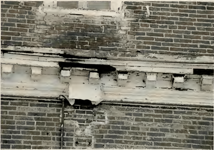
Figure 27 Wood Cornice Deterioration, 1998 Photograph by Author
